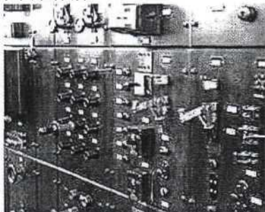
Partial view of the controls and magnetic amp.
